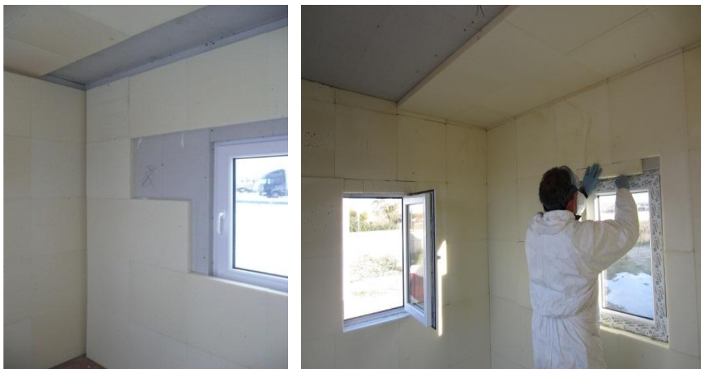
Figure 10 Full panels installation at Warsaw STANDARD (left) and Madrid NANOPCM (right) mock-ups.
