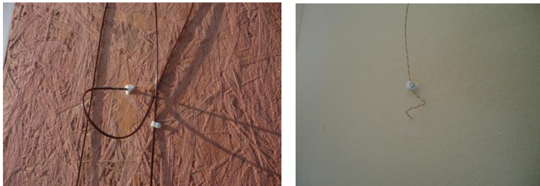
Figure 18 Two examples of thermocouples installation. On the left hand, thermocouple placed on the outside OSB walls at Warsaw NANOPCM mock-up. On the right, thermocouple placed over a PUR panel inside Madrid REFERENCE mock-up (slightly poked on the PUR surface, secured with a plastic flange and stuck with silicone gel).
